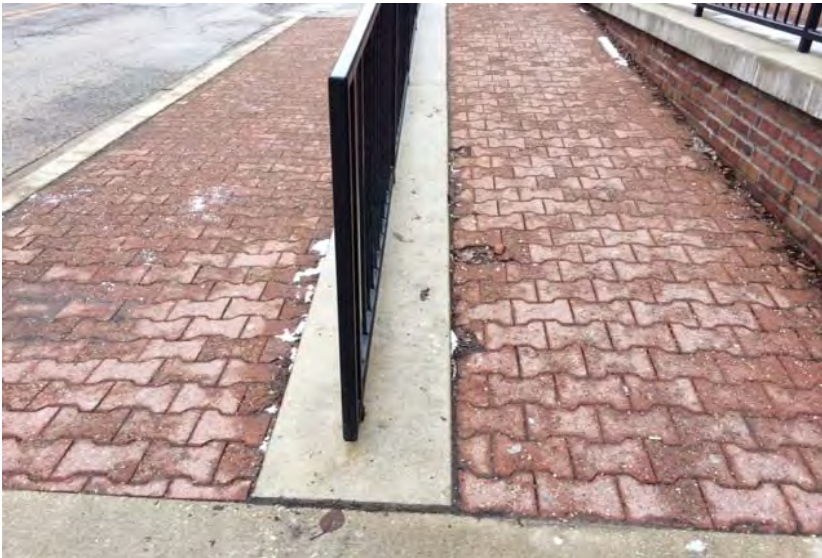
The hardscape along 1st Street shows uneven surface levels.
